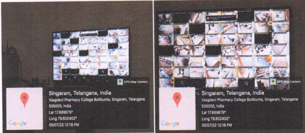
CCTV cameras monitoring
